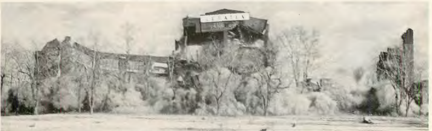
Elevator shaft, in center of building, is separated from building. Structure is collapsing on its foundations.
